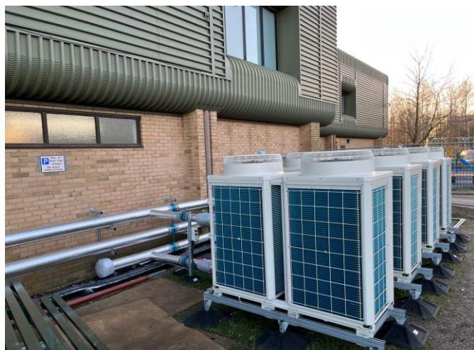
Heat Pumps at Abbey LC
